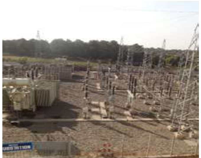
132KVA Sub Station
